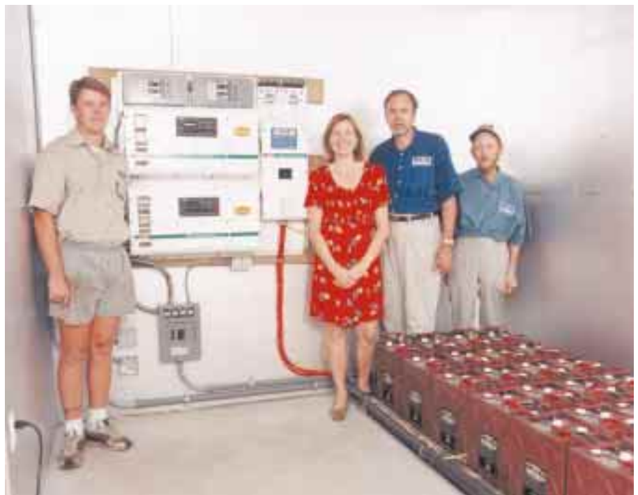
Below: ECS crew members (from left) Jamie Dempsey, Shirley Lane, Tom Lane, and John Ault in the custom built power shed which houses the Trace Power Panel and thirty-two Trojan L-16 HCs.
